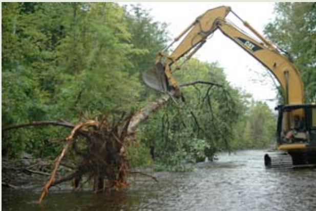
Habitat restoration work such as is being done on the Twin Rivers Farm Project requires the coordinated expertise of many, heavy equipment and lots of materials.
